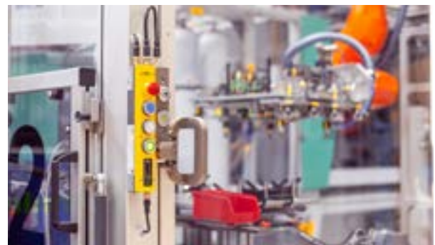
Safety chaining of all safety doors
